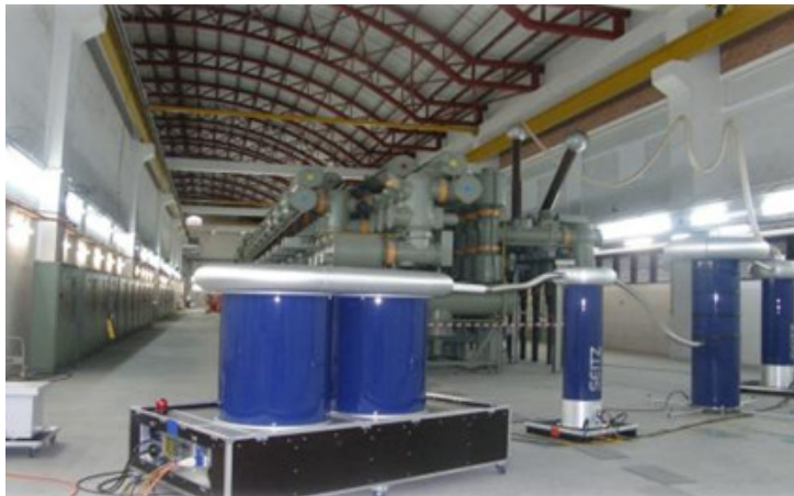
230kV Cables Oscillating Wave Test System
