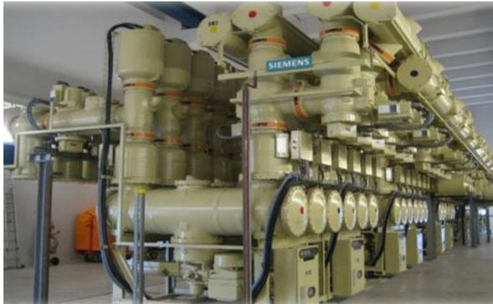
400kV/230kV Potential Transformers Zero Sequence Measurement
